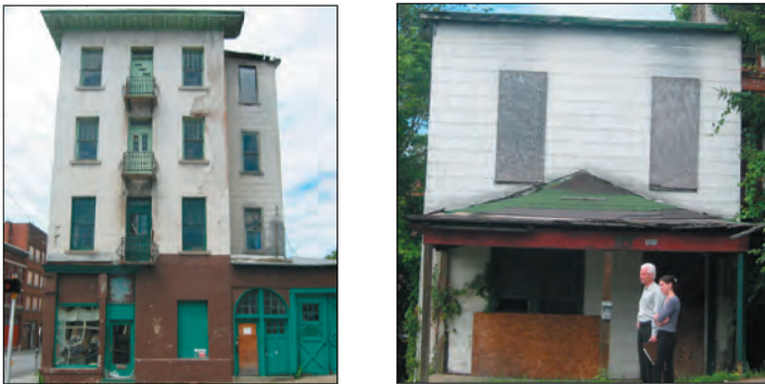
As demonstrated above, many buildings in the RA require comprehensive repairs.
