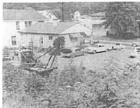
The metal building is needed for the move across the street to Ball Run Plant. It is scheduled off for the relocation.
